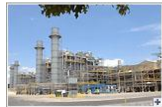
McIntosh Combined Cycle Plant
